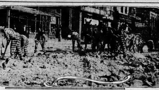
The illustration shows the county convict force at work on the new grade on Whitehall street from Mitchell to Brethren streets. This work was temporarily suspended, but the court desired the illustration at this time as a assurance a speedy completion of the job.
